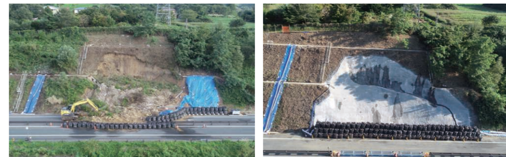
Photo: Minamisanriku Coastal National Highway Office
