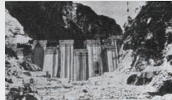
Kansai Electric Power's Kurobe 4th Dam (the so-called Kuro-yon dam) - began foundation construction work in 1960
