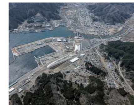
Otsuchi Town, Ando Area Reconstruction Work (Otsuchi Town, Kamihei District, Iwate Prefecture)
