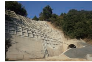
JR Kure Line, Saizaki Area External Disaster Restoration Work (Mihara-shi-Higashihiroshima-shi, Hiroshima Prefecture)
