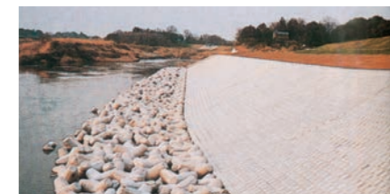
Arakawa River Hirakata Embankment Disaster Restoration Work of the Ministry of Construction (Saitama Prefecture)
