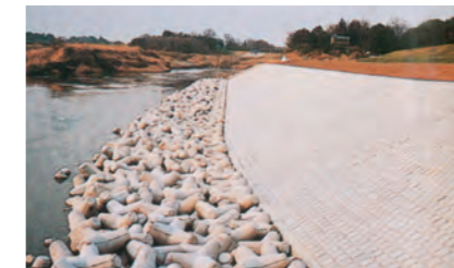
Arakawa River Hirakata Embankment Disaster Restoration Work of the Ministry of Construction (Saitama Prefecture)
