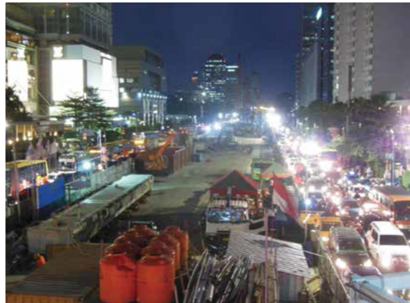
Chemical grouting for corner reinforcement of diaphragm wall corner for the station building
